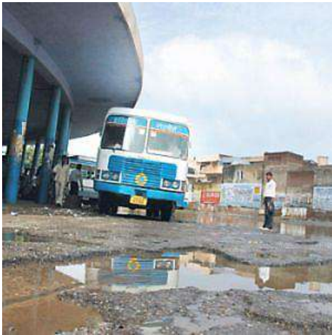
Figure 2: Dilapidated Bus Terminal, Gurgaon (hotgurgaon.com)
